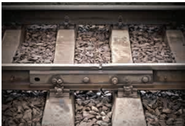
Figure 1.1 Gap in railway track
